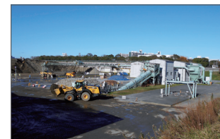
General view of the Nakagawa Construction-Generated Soil Improvement Plant
