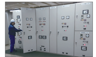
Survey for equipment reconstruction at sewage treatment plant and pumping station (survey of the current condition of electrical equipment)
